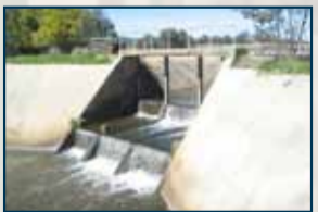
A slot board barrier on Logue Brook
