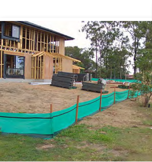
A sediment fence installed around a new home site to improve sediment capture. Source: Healthy Land and Water and Brisbane City Council
