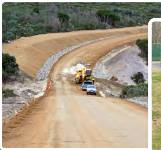
Stabilisation of newly-constructed batter and table drain using coir matting and rock armouring as part of road works construction. Photographer: Matt Coppen, Main Roads WA.
