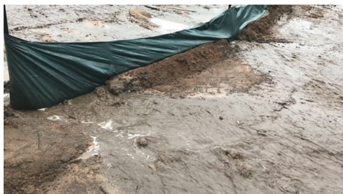
Sediment fences are ineffective if not implemented correctly
