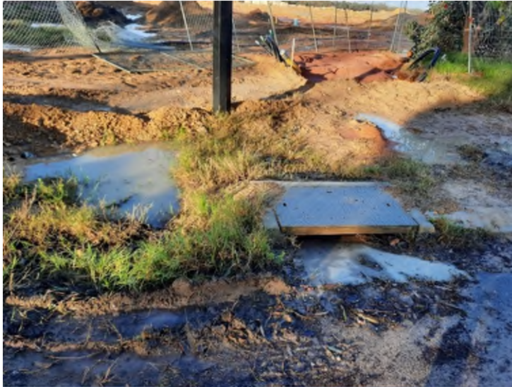
Figure 5: Sediment run-off from a development site entering a drain. Image source: Bronwyn Scallan, Perth NRM
